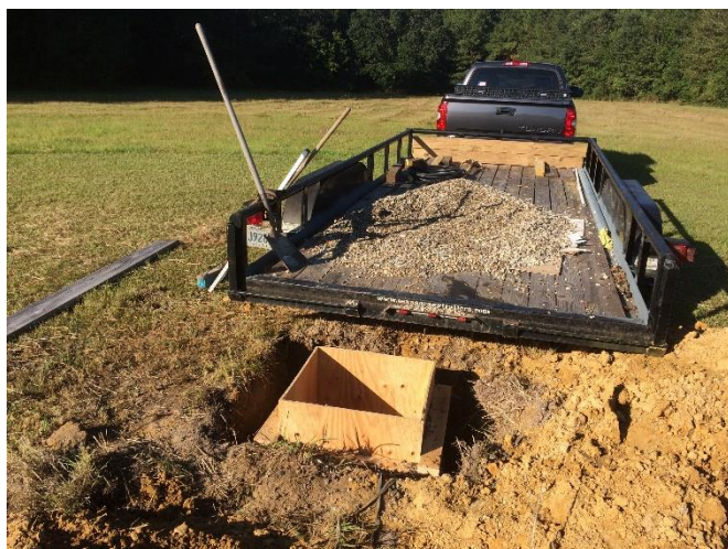
The hole is dug, 2-foot square by 4 feet deep formwork is in and rock for drainage is being placed.
