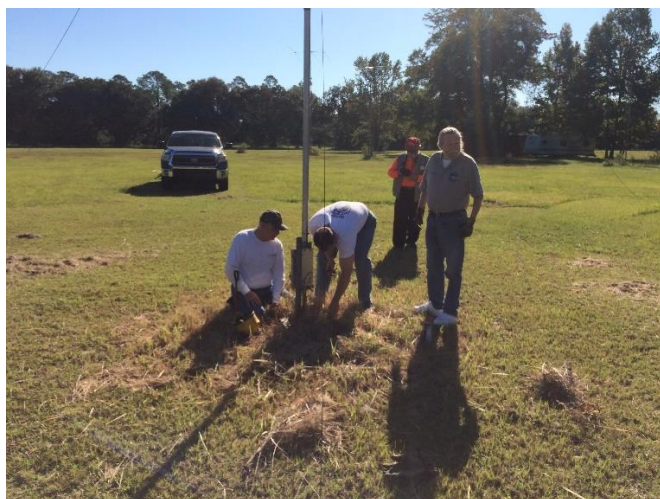
Locating the radials at the old antenna prior to taking the antenna down.
